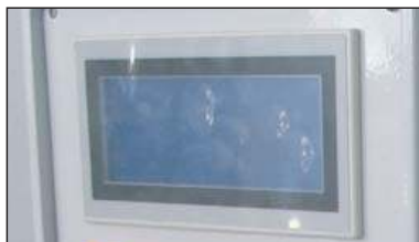
PLC control touch screen panel
