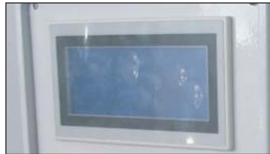
PLC control touch screen panel
