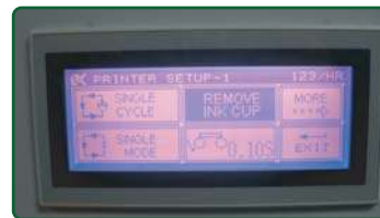
PLC control touch screen panel
