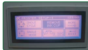
PLC control touch screen panel
